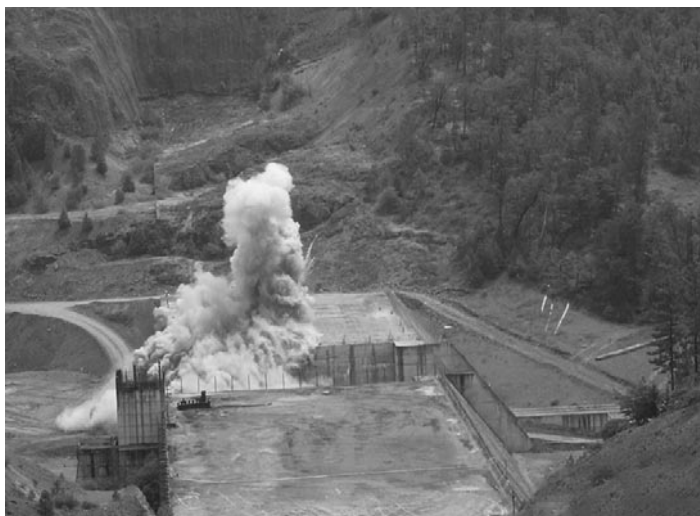
Officials began the process of notching the Elk Creek Dam with a July 15, 2008 explosion. The job will be completed this fall. Photograph by WaterWatch of Oregon
